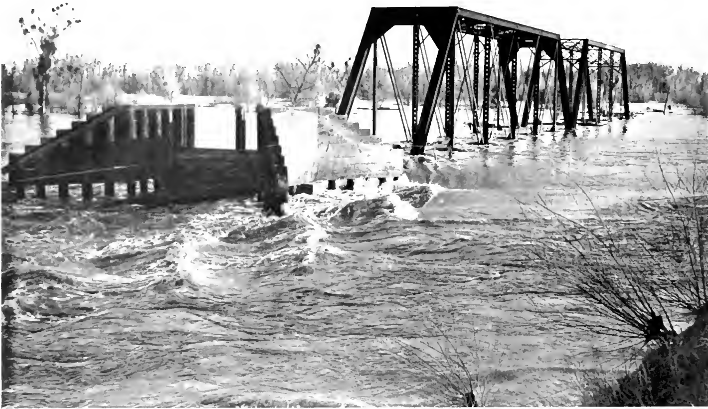
Portion of railroad bridge span damaged by February break of Feather River levee in Reclamation District 803
